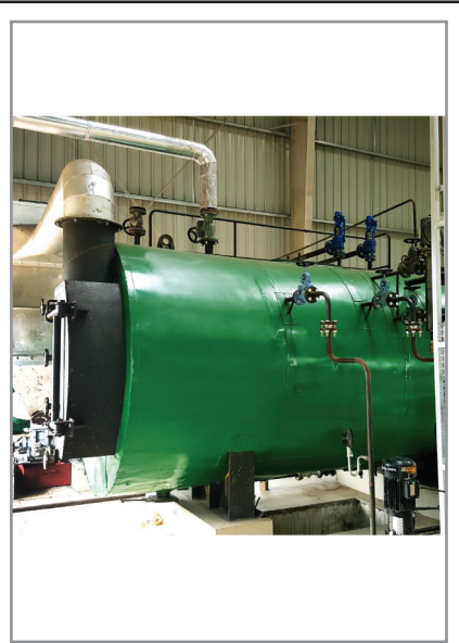
CASHEW NUT HMT BOILER
